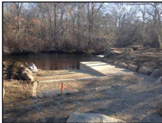
Cronan Universal Access Boat Launch (left) and Fishing Pier (right) during construction
