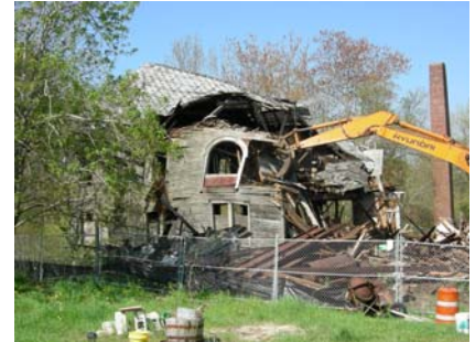
The former Knowles Mill in Shannock, demolished in May, will become the site of a park and portage on the river.
