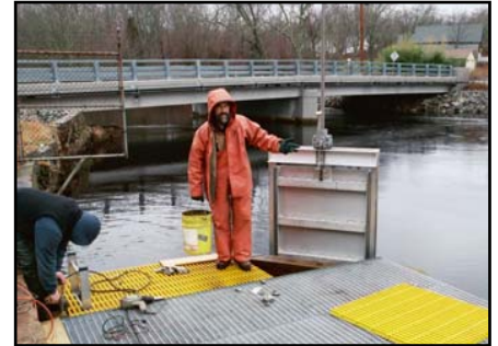
Workers for RI Department of Environmental Management install a new gate and platform at the Potter Hill Fish Ladder on the Pawcatuck River.
