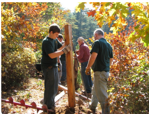
Eagle Scout volunteers from Troop 1 Charlestown work together to rebuild the split rail fence at Browning Mill Pond.
